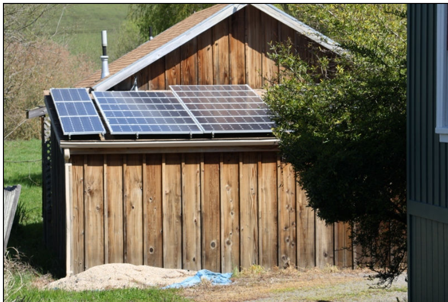
Figure 26 - Solar panels discretely placed on an accessory structure
