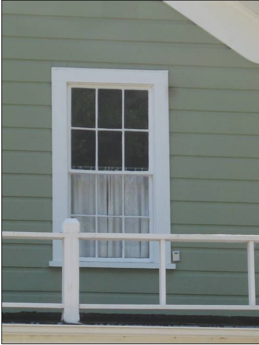
Figure 12: Hind's Hotel, 306 Bohemian Highway. The building has historically been clad in painted, wood shiplap siding.
