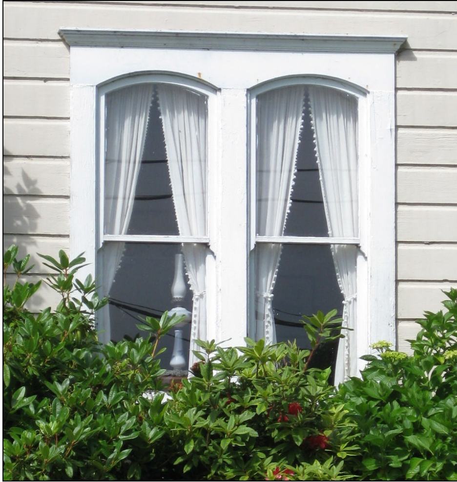
Figure 15: Residence, 520 Bohemian Highway. Although the original windows were likely wood, two-over-two, double-hung windows, the replacement windows are paired, narrow in width, and have a segmental-arched, upper sash. Therefore, they maintain the original windows' historic shape, operation, details and finish.
