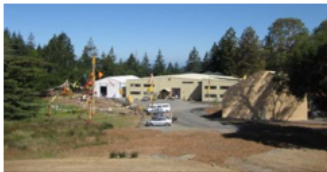
The printing operation was definitely a factory... The 21,234 square-foot printing factory at Ratna Ling Retreat in 2009.
