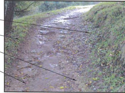
TRAIL IN NEED OF RECONSTRUCTION
